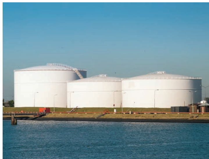
Figure 21.9 Bulk petroleum storage tanks. Fuel tanks often support microbial growth at oil–water interfaces.
